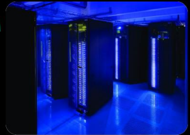
High Performance Computing Facility (HPC)
